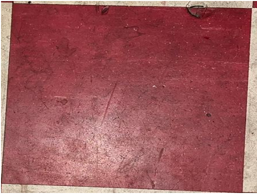
514-1 Adhesive 9"x9" Floor Tile/Red (3% Chrysotile) Mastic Interior Bedroom B (Approx 55 sq ft)
